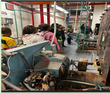
Student Green Team (SGT) members are in the boiler room learning about the different functions.
