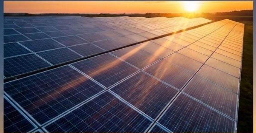
Solar Farm at Sunset.
